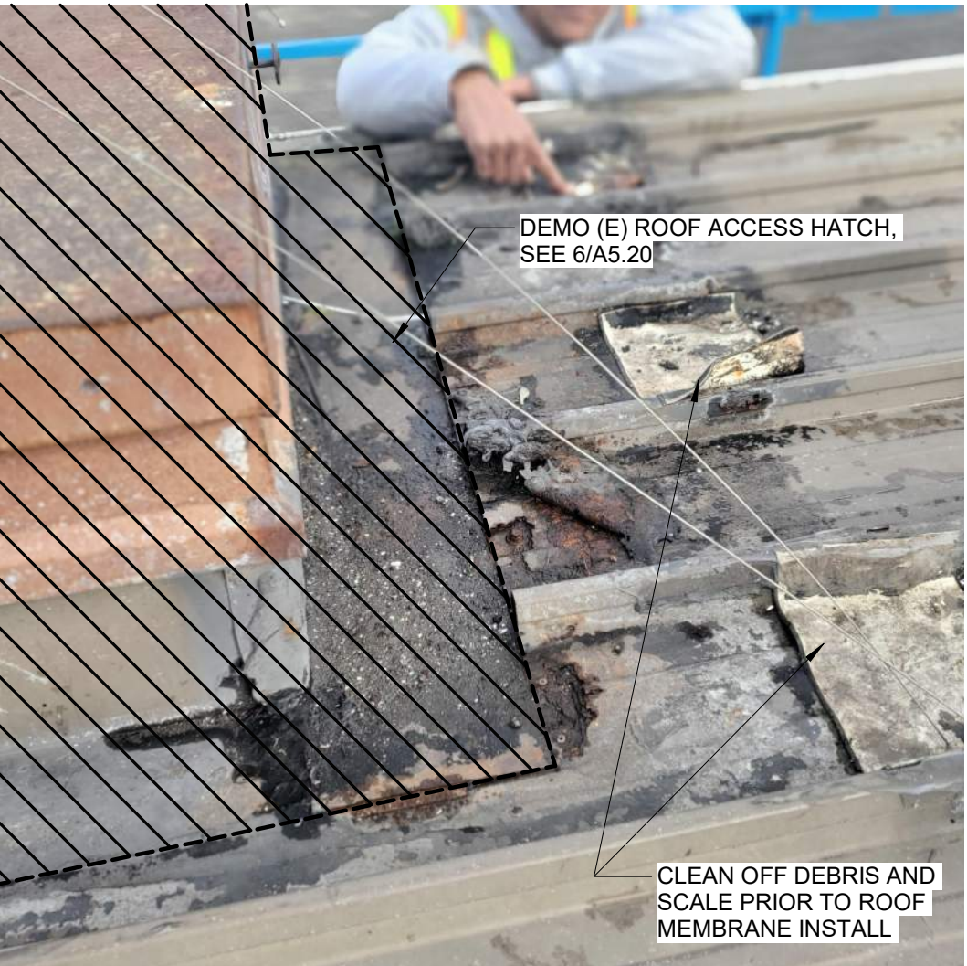
8 AD9.20 RUSTING AT ROOF HATCH NTS
