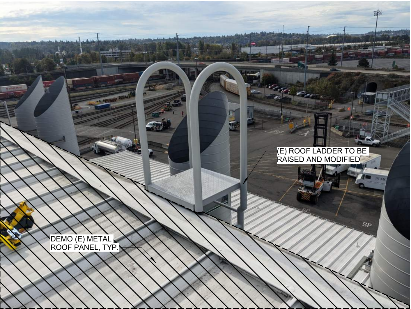
3 (E) ROOF ACCESS LADDER AD9.10 NTS
